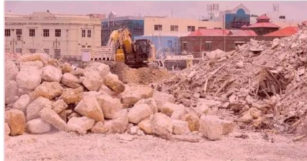
A bulldozer was onsite on Thursday when the Sunday Sun passed. A decision was made to salvage the stone blocks from the demolished structures for use in the new buildings. (Picture by Shanice King.)
